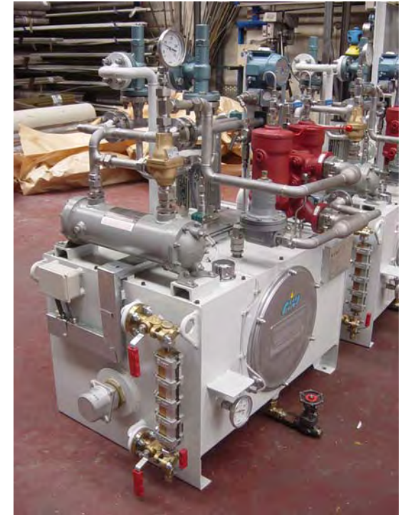
Lube Oil Units, C.T. Elm Road – USA, Bechtel
